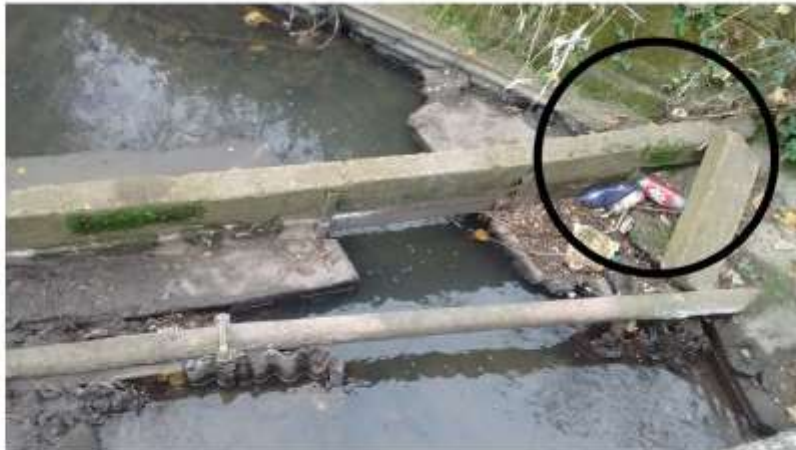
Figure 4: This image shows the two structures comprising site 2, the black circle highlights where the weir has been joined to the bank walls at one side.
