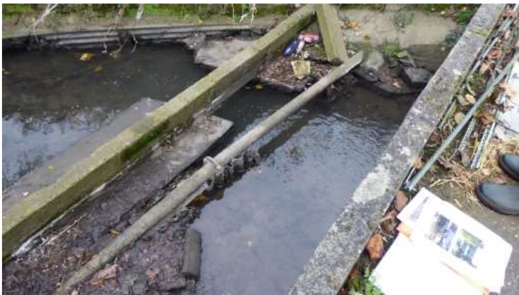
Figure 1: An image of Site 2, the second weir at The Dene.
