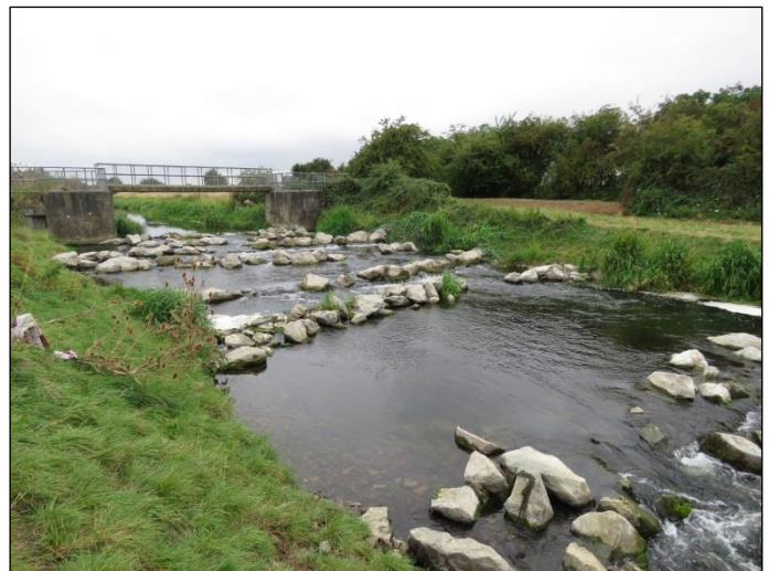
Fig 2. After – the completed Aubourn Rock Ramp. Fish and eels can now pass freely upstream and downstream.
