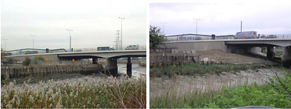
Figure 3.3: Land Nr 13: View of frontage before works (from Cuckholds Haven), and after retreat of flood defence and creation of intertidal zone (EA Archive).
