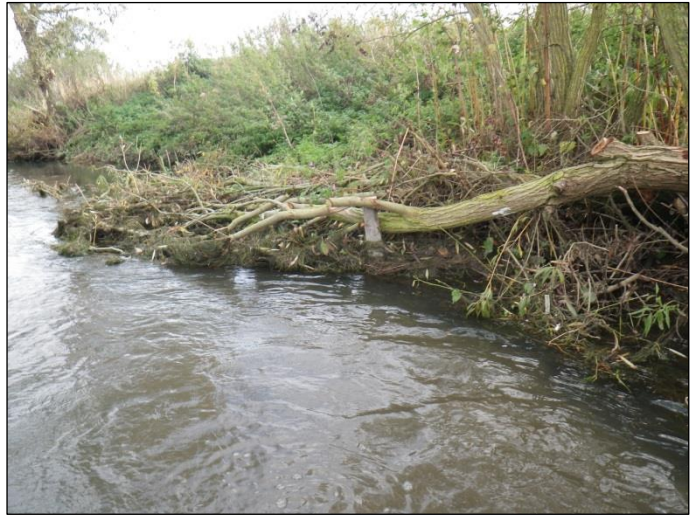
Fig 2. Hinged and pinned riverside tree with added brushwood to narrow the channel and trap fine sediment. (Syston)
