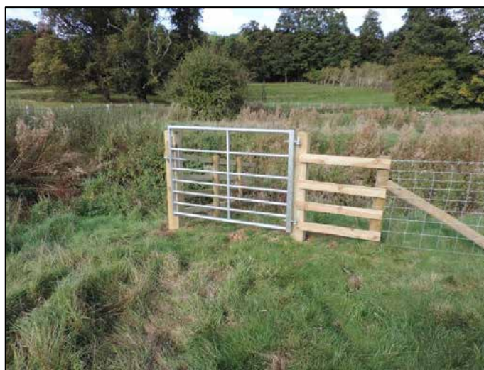
Fig 21. A hand gate installed at the end of a long run of fencing. Note the reversed stock netting with the larger mesh at the bottom to allow better access for pheasants. (Phase 1)
