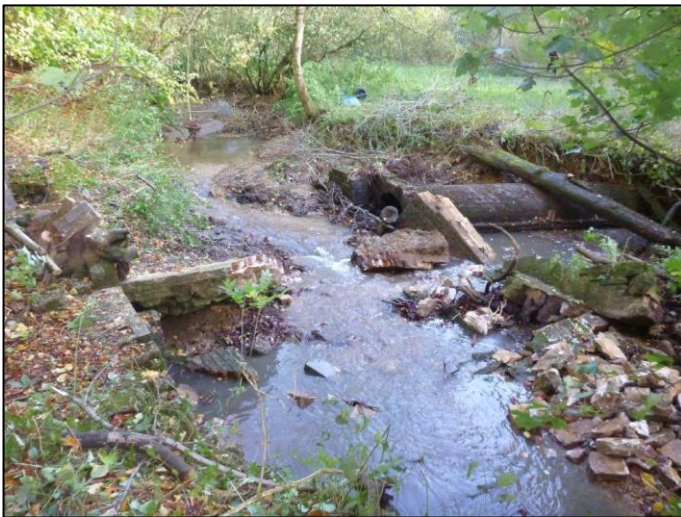
Fig 24. View upstream immediately following the removal of the central section of the weir which restored the flow to the main river channel (October 2014).
