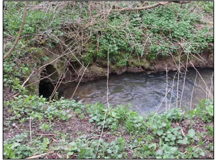
Fig 23. The weir bypass culvert in April 2014 before the removal of the weir crest. The culvert is redundant now that the weir crest has been removed.
