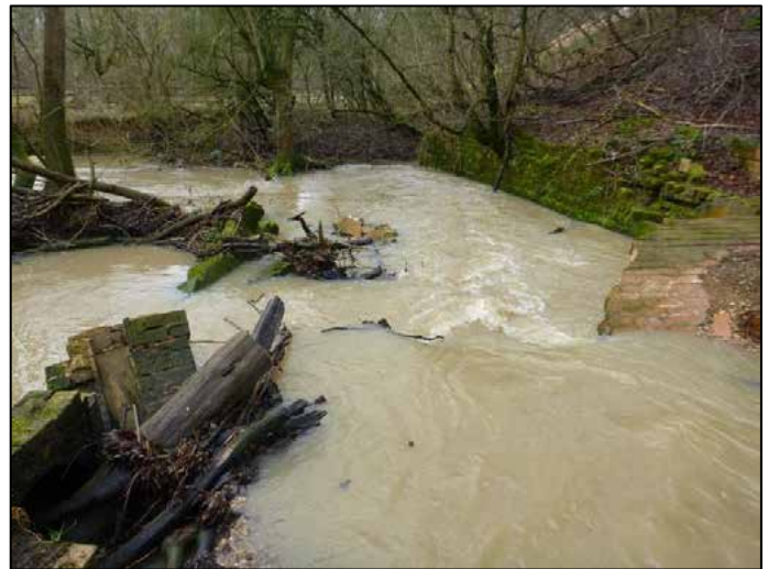
Fig 25. Subsequent high flows through the breached structure (February 2015.).
