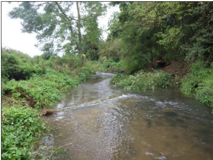
Fig 11. Single flow deflector in conjunction with brushwood mattresses demonstrating how the flow is modified (Phase 2)
