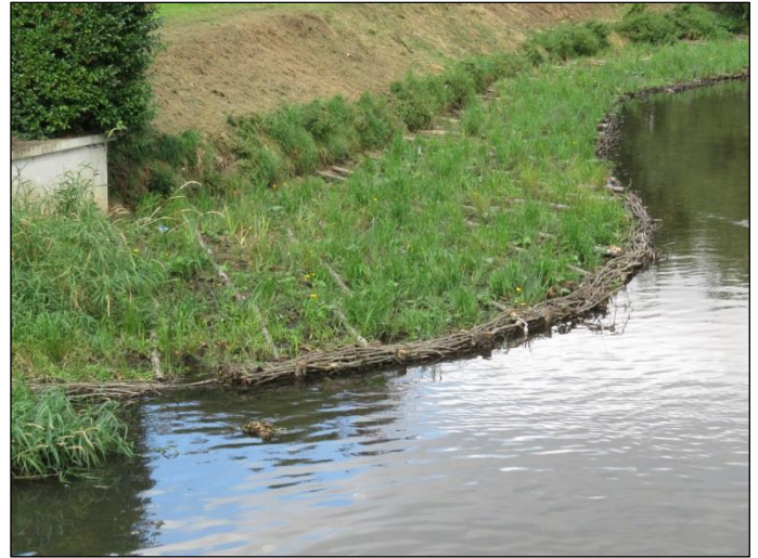
Fig 4. The soft berm, edged with faggots, infilled with sediment excavated from the river and topped with pre-planted coir.
