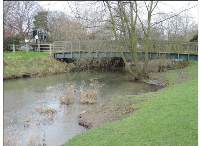
Fig 2. Before (December 2014). Upstream of the Belton Lane footbridge the river bank was heavily-eroded (also see Fig 7).
