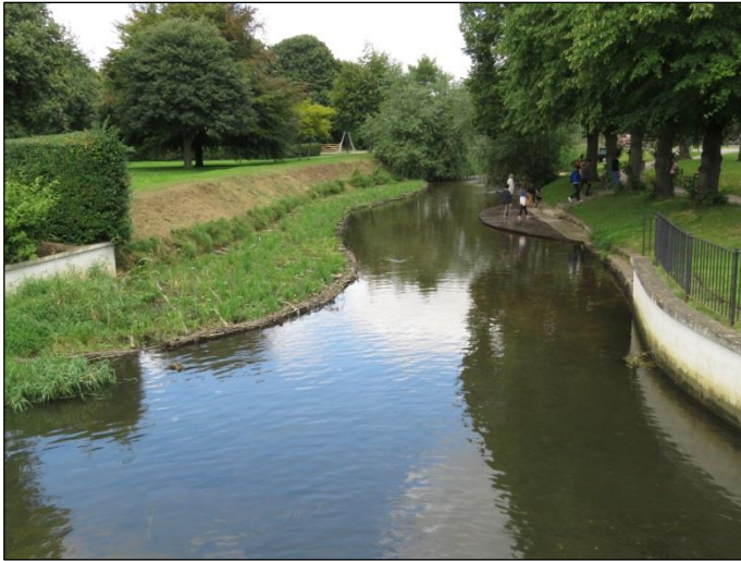
Fig 3. The newly restored channel. The planted berm on the left bank narrows the river and softens the hard bank, while park visitors enjoy the new access decking.
