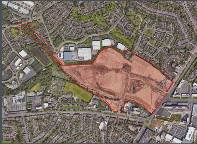
2022 Longbridge West Site – Construction works for the renaturalisation of the River Rea being undertaken
