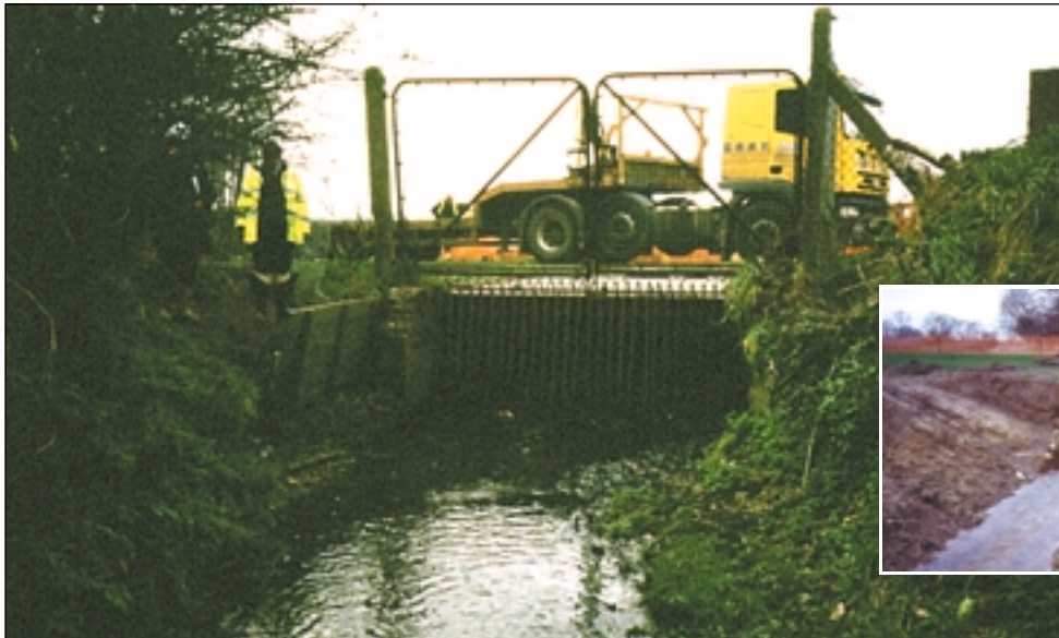
View of headscreen prior to removal
