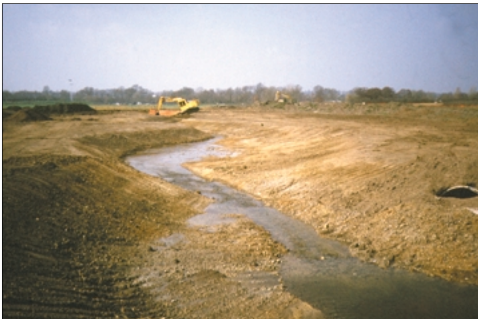
Looking downstream at the shallow bank slopes. The severed culvert still visible
