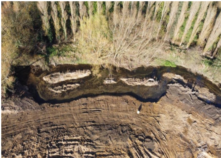
Fig 5. Post works showing channel widening, gravel riffle, island and point bars installed and multiple threaded channels installed with woody material secured in the river and on floodplain..
