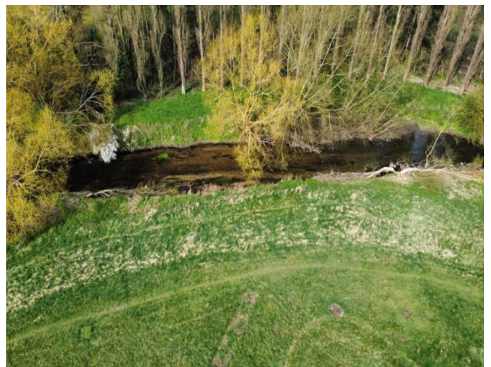
.Fig 4 – Pre restoration works aerial shot showing embankment in situ and hinged trees in channel.
