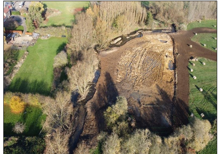
Fig 2. Post works – (Nov 2021). Flood embankments removed from floodplain and part of floodplain lowered by 30cm with ponds and scrapes added to increase habitat types. The floodplain is terraced with a lower more frequently inundated landscape close to the river and then gently rises up towards the valley sides which will inundate less frequently but in higher flood event magnitudes..
