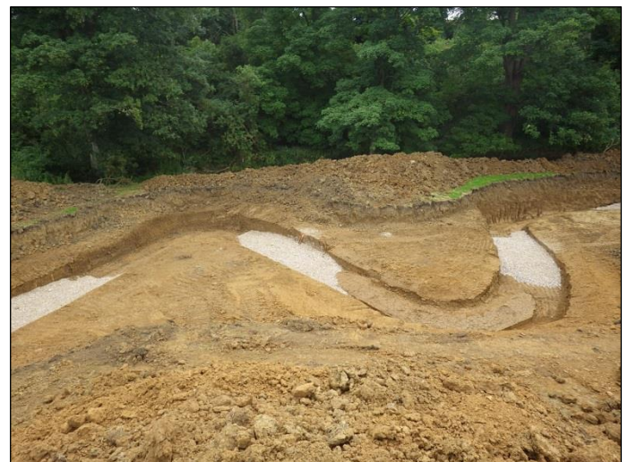
Fig 17. Gravel was introduced at predetermined locations while the channel was still dry to form the pool- riffle sequence
