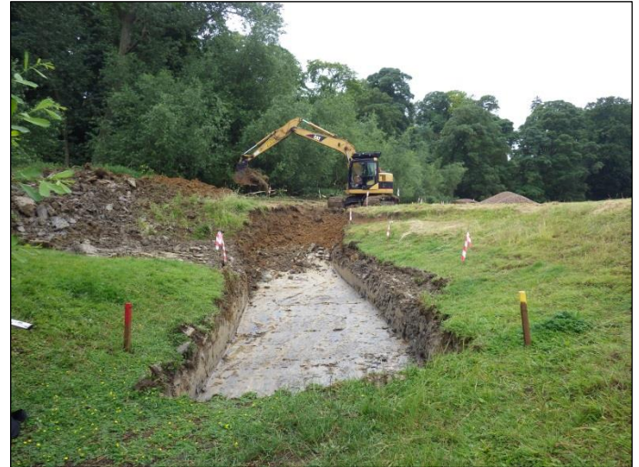
Fig 15. Start of the channel excavation following pegging out of the planform on the ground
