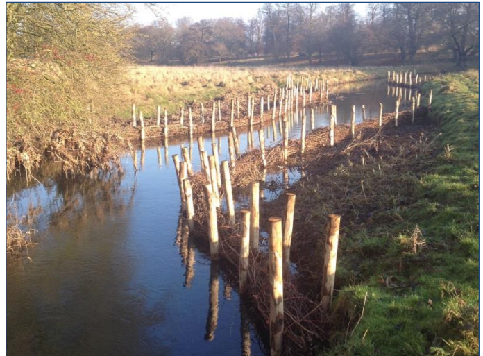
Work in progress on a faggot-fronted berm to trap fine sediment, narrow the channel and speed up the flow
