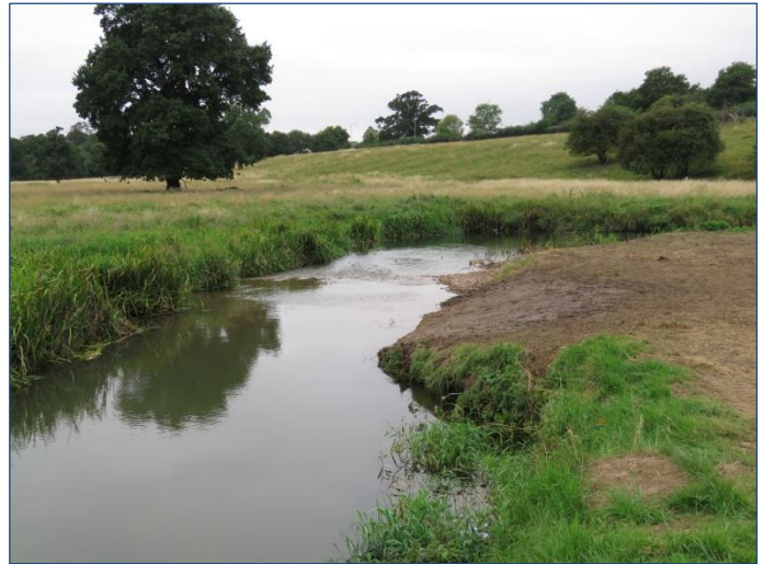
After – New gravel riffle created to speed the flow and bank lowered to improve the floodplain connection
