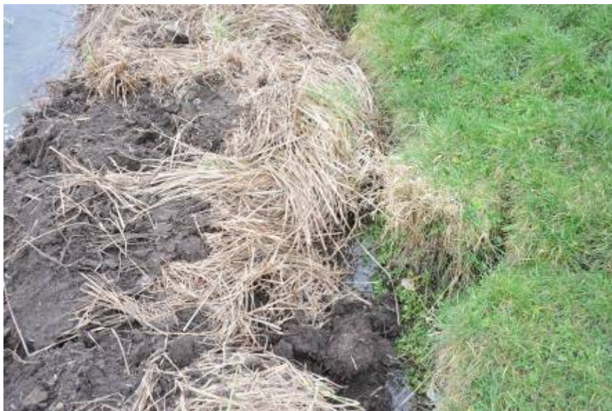
Example of retained gap between in-fill to narrow the channel and the existing bank
