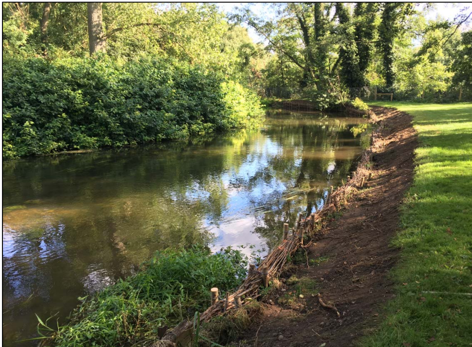
Steep banks suffering erosion has been re-profiled to encourage marginal vegetation to establish.
